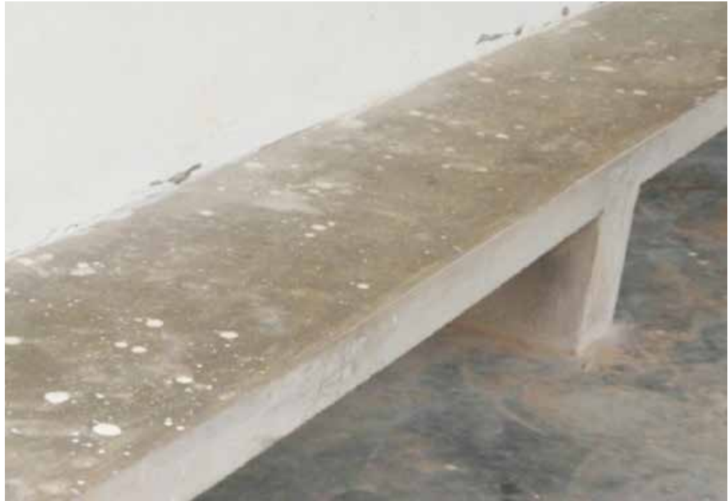
Above, cracks along the joint of a concrete bench.
