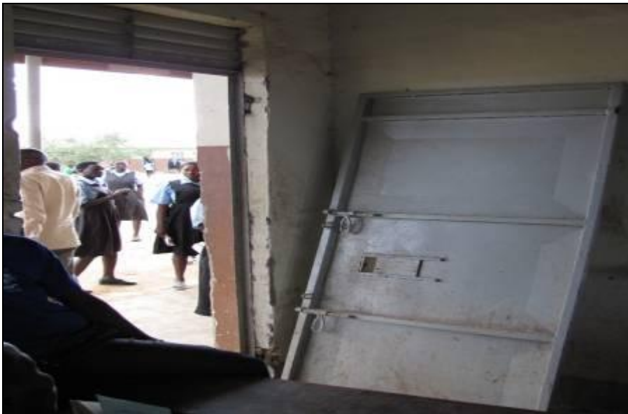
Picture 6: A picture of Nadunget Seeds School in Moroto District show total failure on fixtures and fittings. This door is totally out of its position.
