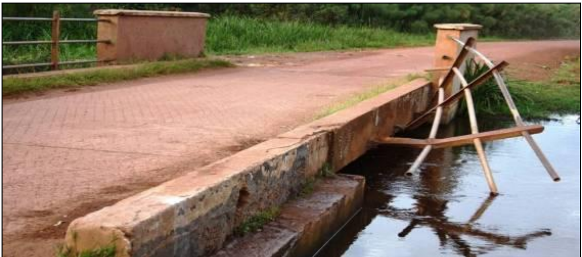
Picture 39 A broken bridge structure not replaced within the stipulated time frame. This is a danger to the road users.
