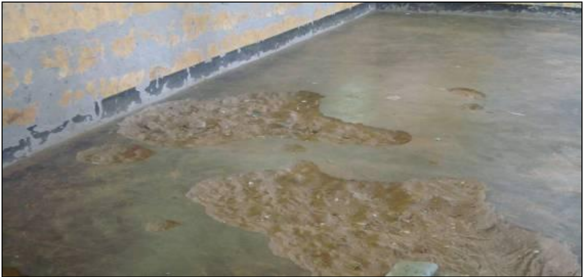
Picture 11: A poorly constructed floor and plaster of a classroom at Opeta Primary School in Apac District, barely two years after construction.
