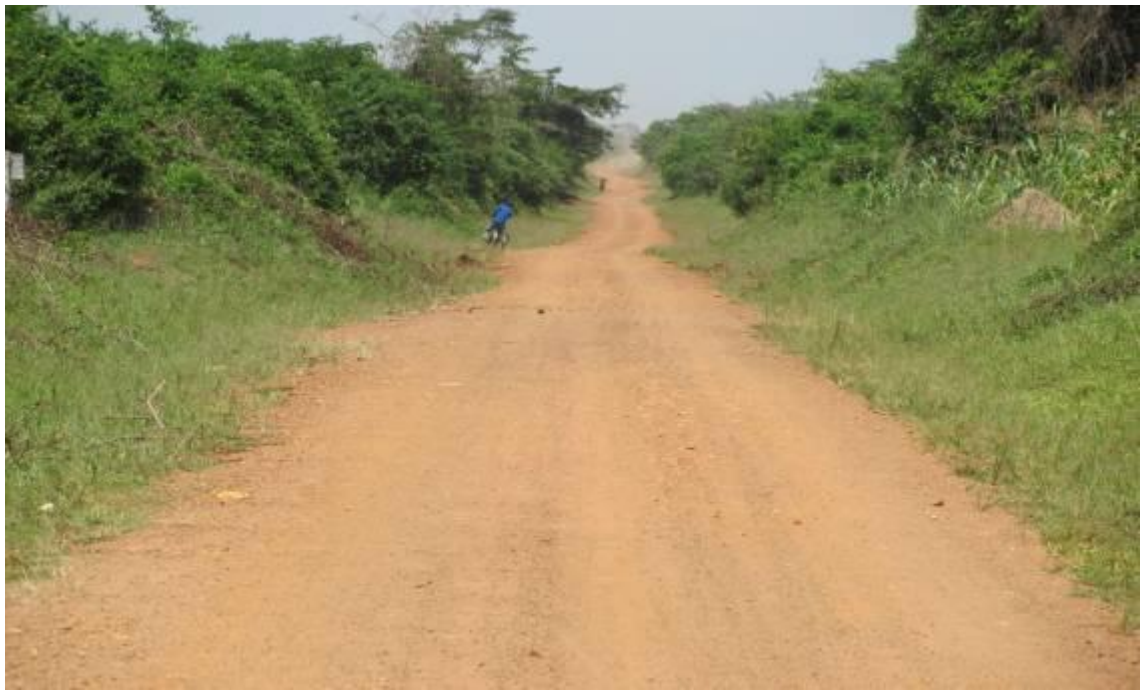
Picture 29: A section on Km 11+800 (Kamuli - Namasagali Rd) has a narrow right of way as a result of overgrown grass on the shoulders.
