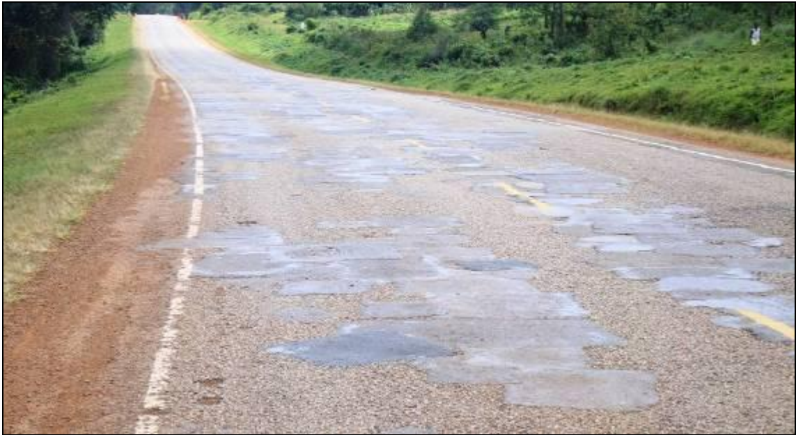
Picture 25: A section on Fort-Portal Kyenjojo road with over-patching that did not have lasting impression since the road structures had substantially failed. UNRA should have established the cause of the distress and come up with the most appropriate intervention measure instead of spending much time and money on patching.
