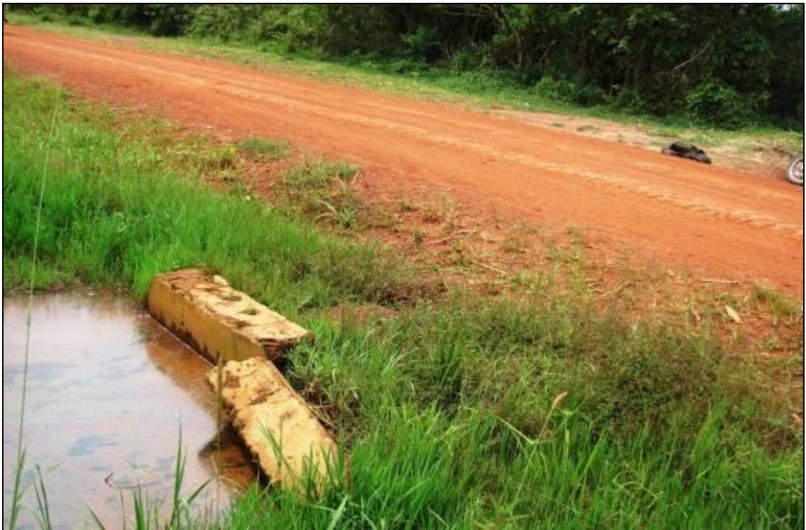
Picture 33: An example of a clogged culvert bridge with broken head walls on Ngeta-Puranga road, as a result of lack of maintenance.
