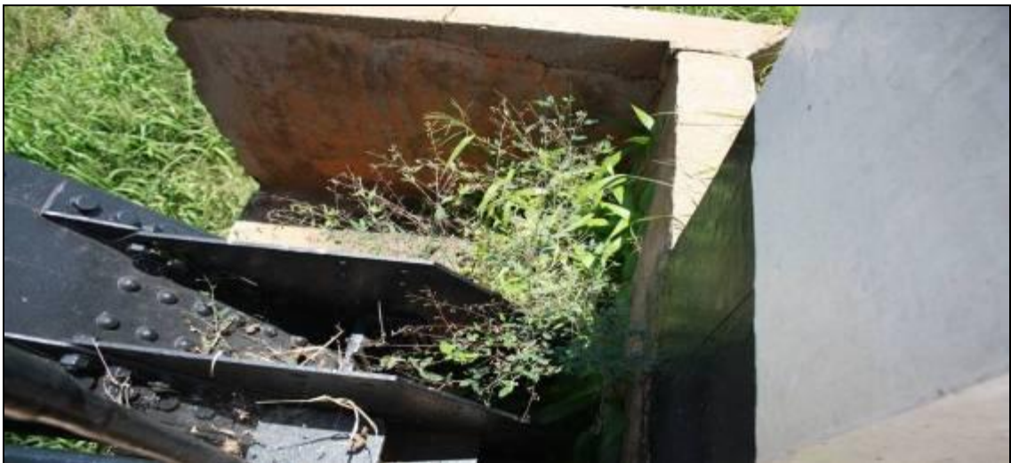
Picture 36 Bearing position on ORA Bridge in West Nile clogged with grass. Greasing was not done on this bearing. This weakens the bridge and shortens its life.
