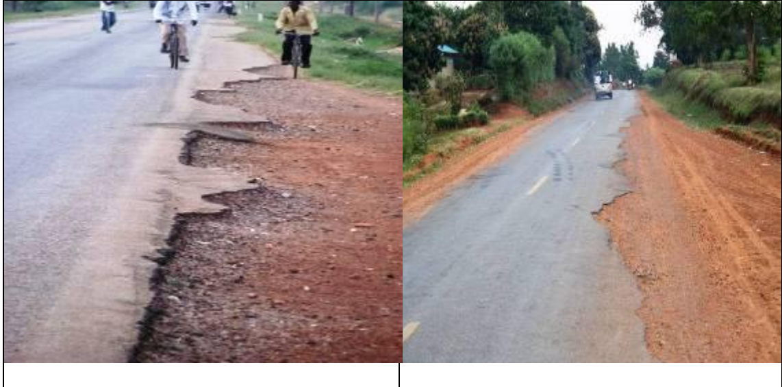
Picture 31: section on the Tororo-Malaba Rd on the left above that is slowly eating away towards the carriageway and on the right a section on Mbale-Sironko Rd that has edge of mat failure up to the road centerline.
