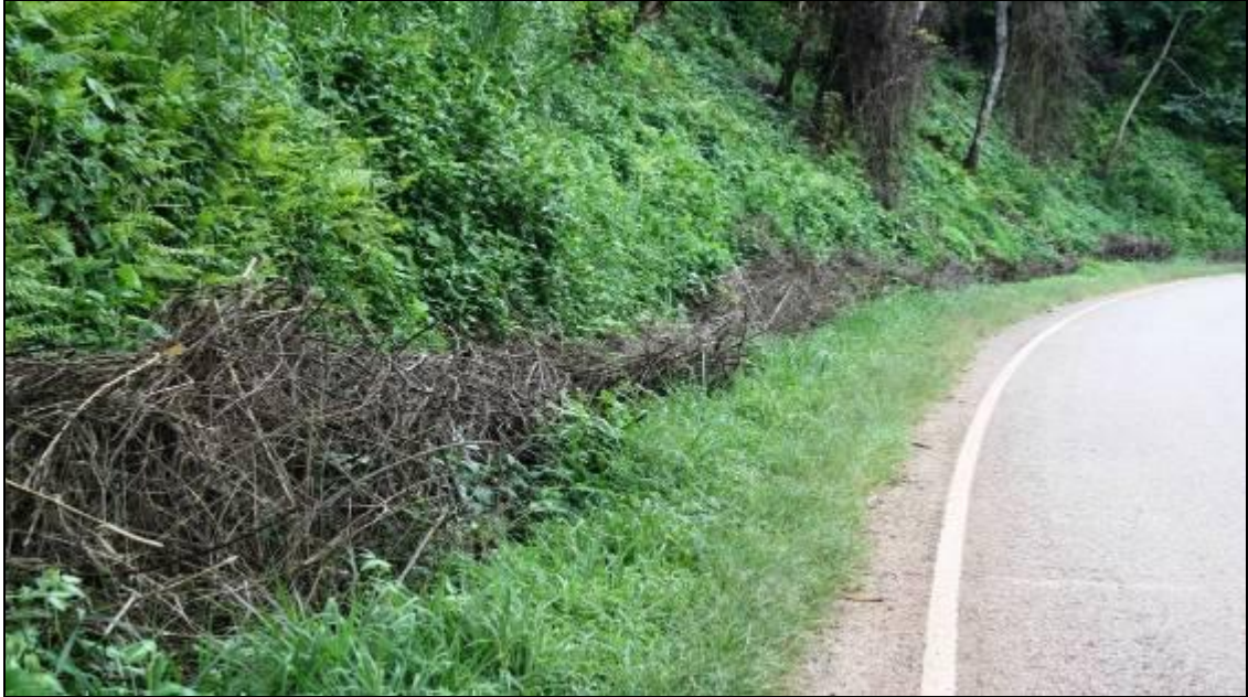
Picture 28: An example on a section of Kyenjojo-Fortportal road where grass was cut but not disposed of as per specification within the manual. Grass was instead dumped in the drainage, blocking running water.
