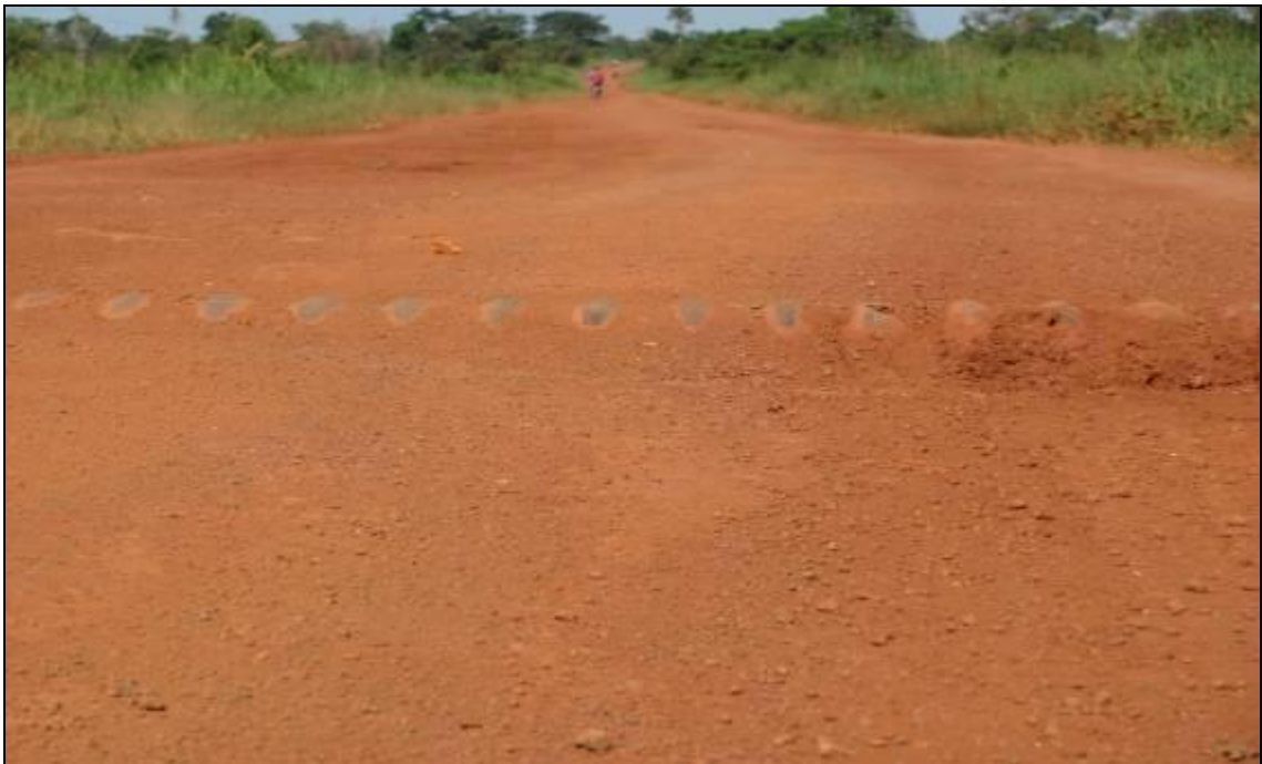
Picture 22: A section on Lira-Aduku Road at Banya swamp km 11 with visible inadequate gravel cover that exposed the culvert. Such a culvert is a potential danger to motorists. The culvert stands a danger of being blocked by gravel as evidenced by the developing holes.
