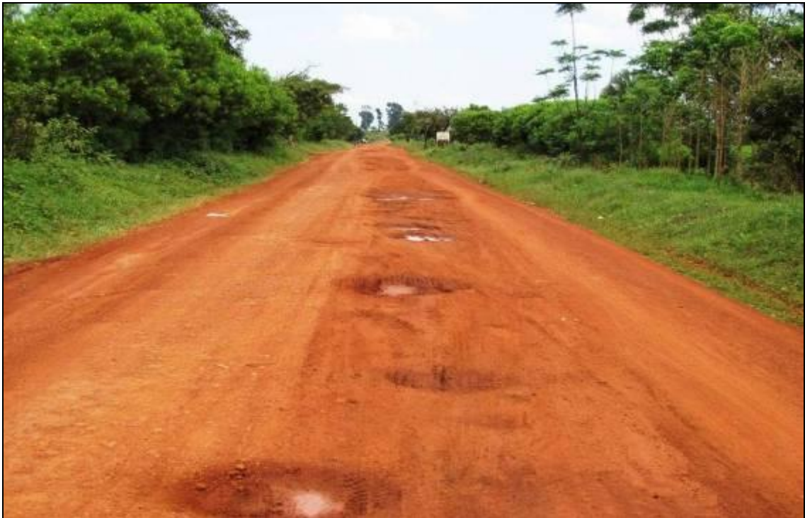
Picture. 35 Another spot on the same road Ngeta-Puranga. The road lacked adequate super elevation and therefore, failed to drain water into the ditches.
