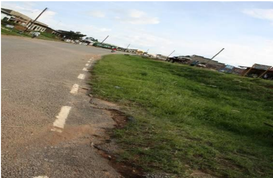
Picture 27: An example of ungraded/ un-mowed road edge on km 17 Mbarara Ibanda road at Igorora Town Board. The water had been diverted onto the carriageway and had eroded the.
