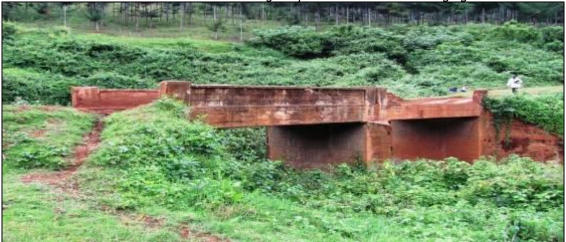
Picture 38 Siti Bridge that was constructed in 1953 with knocked down guard walls that were never replaced. Notice the over grown vegetation underneath the deck that blocks free flow of the river.
