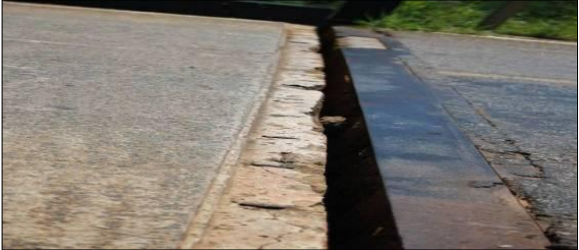
Picture 37 Road not shaped to match bridge deck on ORA Bridge. This is a big danger to the motorists because it could lead to bursting of tyres due to constant banging of the ream.
