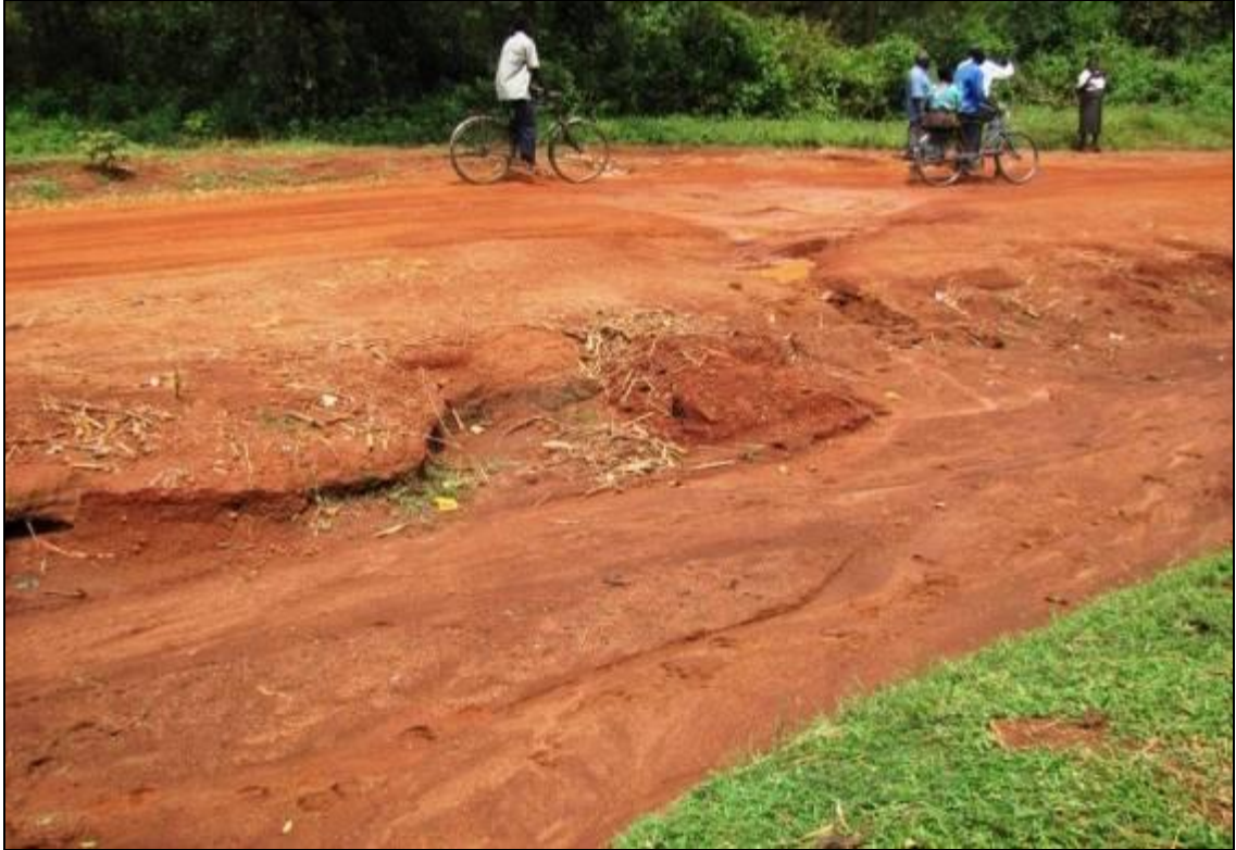
Picture 34 A spot on Ngeta–Puranga road. This road located in Lira has very poor cross section. Consequently, drainage and overall driving conditions are bad.
