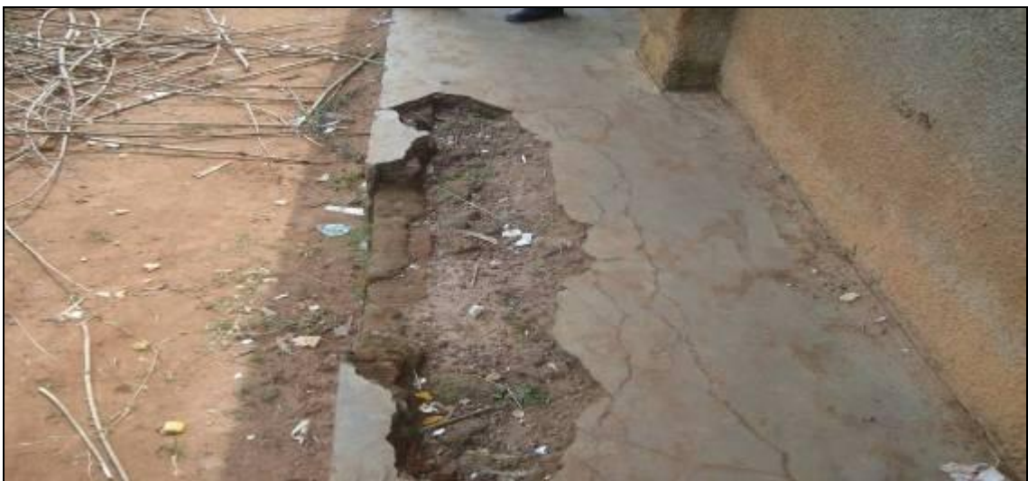
Picture 12: A splash apron on the same building (Opeta P/S) that had completely fallen apart, a sign of poor workmanship and use of inferior materials.
