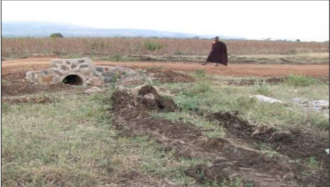
Picture 13: A poorly constructed culvert on Turutuko-Apeitole road in Moroto District where direct procurement was used and the contractor failed to complete works.
