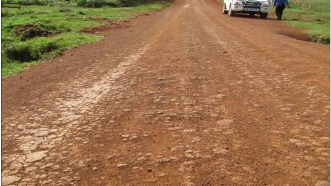
Picture 23: A section on Kapchorwa-Kapkwata Road which has a rough riding surface as a result of compaction done under excessive moisture condition and loss of gravel.
