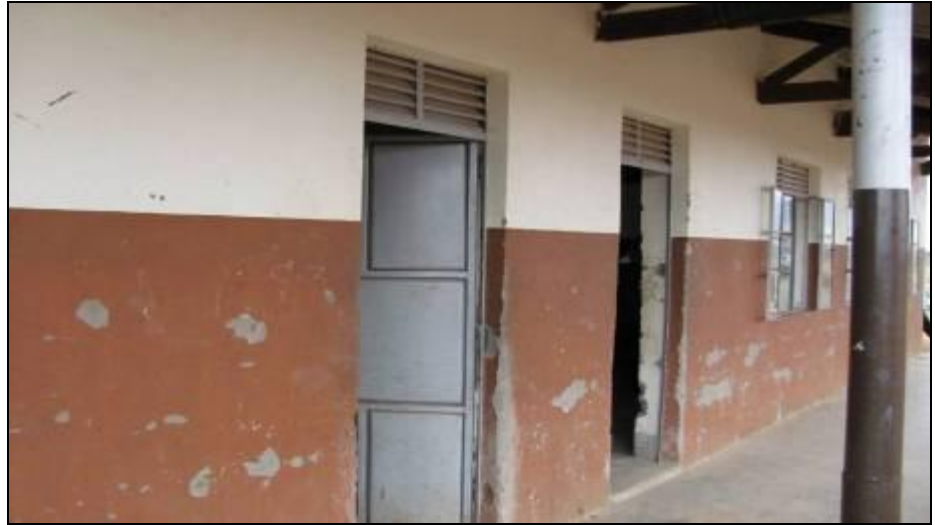
Picture 7: Shoddy works on walls and paintings of Nadunget Seeds School in Moroto District
