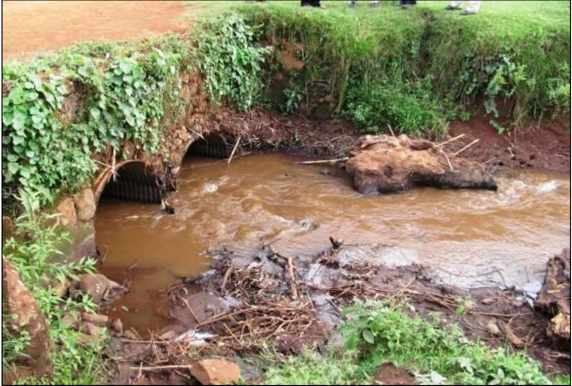
Picture 32: An example of a clogged culvert bridge on Kapchorwa Kapkwata road, as a result of lack of maintenance. This road could fail if debris is not cleared before the next heavy rains.
