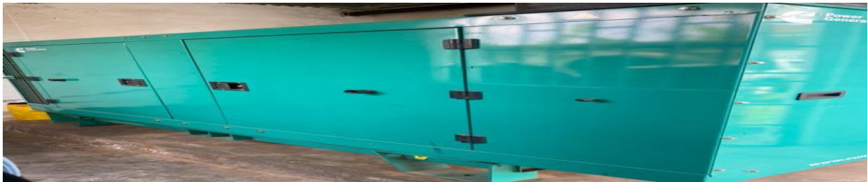
Stand by generator in excellent condition
