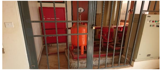
Fire suppression system
