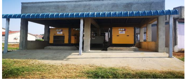
Generators for the new building (CIP)
